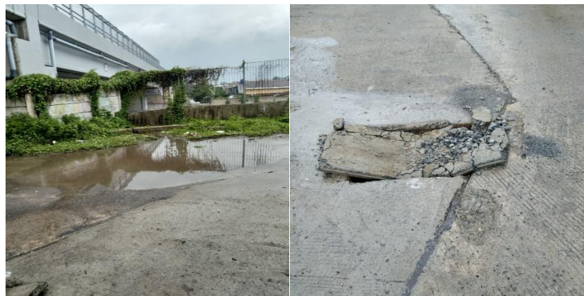
Figure 7. The Flyover Underpass Was Flooded and Damaged
