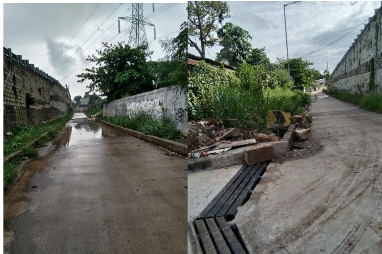
Figure 6. The Road North of the Flyover is Flooded and Slums
